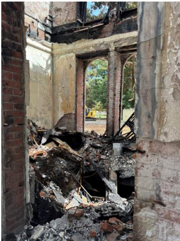
08: Interior debris and conditions, 09.09.25.
