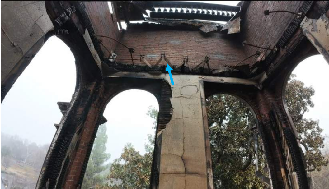
23: Bidwell Mansion tower seismic retrofit remains.
