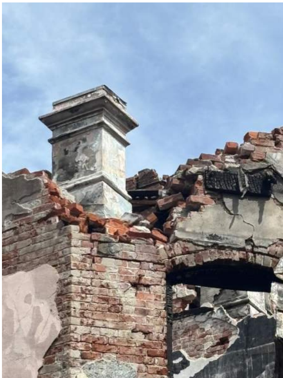
14: Exterior conditions- damaged brick, 09.09.25.
