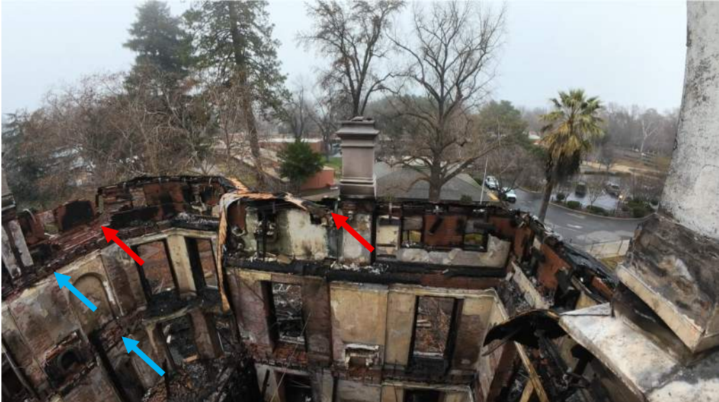
19: Bidwell Mansion interior looking North towards the Visitor Center parking lot. Red arrows indicate sections of third story walls damaged by the collapsing roof. Blue arrows indicate where collapsing floors damaged the walls.
