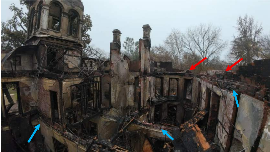
21: Bidwell Mansion interior looking East. Red arrows indicate sections of third story walls destroyed by the collapsing roof. Blue arrows indicate where collapsing floors damaged the walls.
