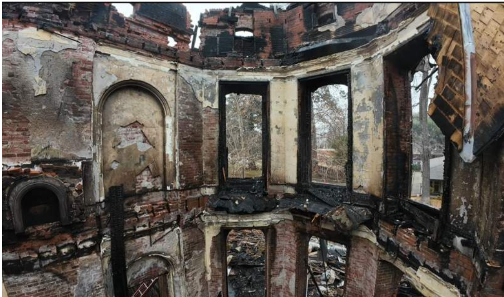
26: View of typical pockets in brick wall where wooden framing has collapsed.
